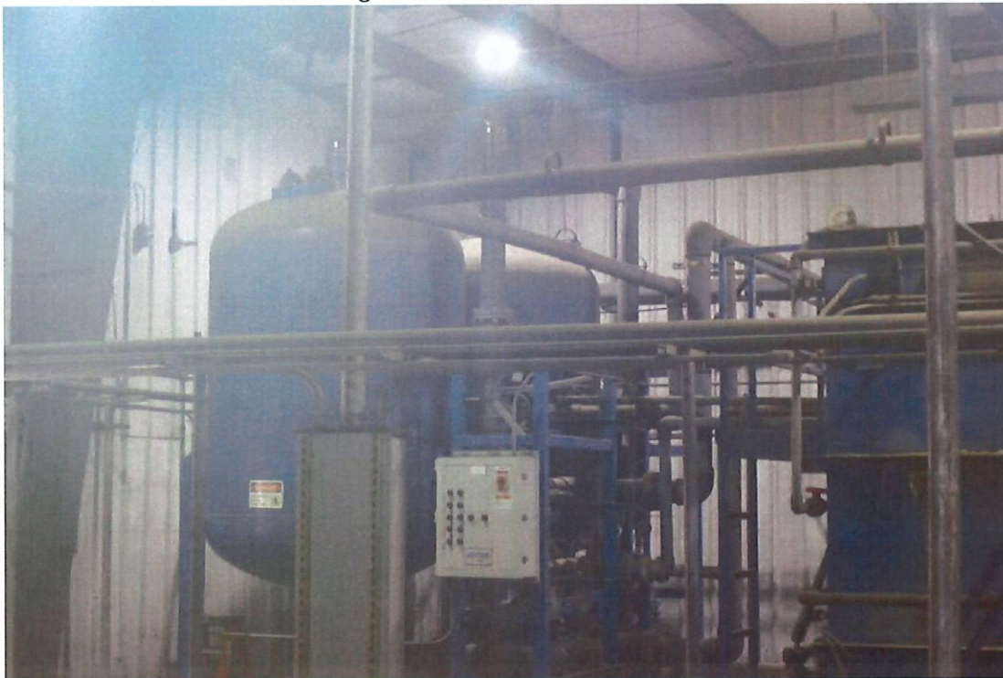
Photo 3: GAC units after existing clarifier.
