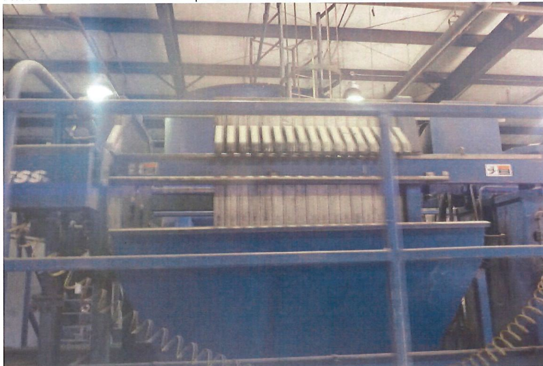
Photo 4: Plate and frame filter press.
